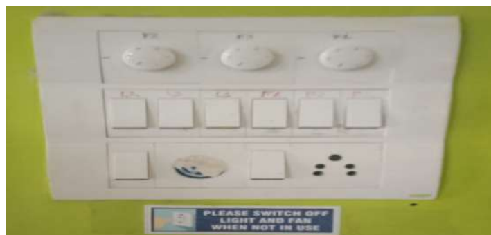
Figure 4:- Signage on Switch Boards
